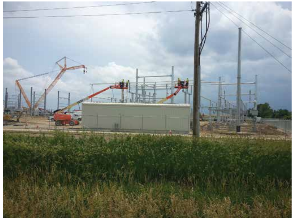
Construction continues at the Iowa Fertilizer Company near Wever. Northeast Power is working with Access Energy Cooperative crews on building the substation that will provide power for the plant.
